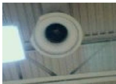
Then, they fell down barely missing the students...
