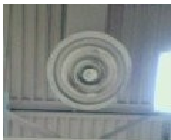
First there were old vents....
